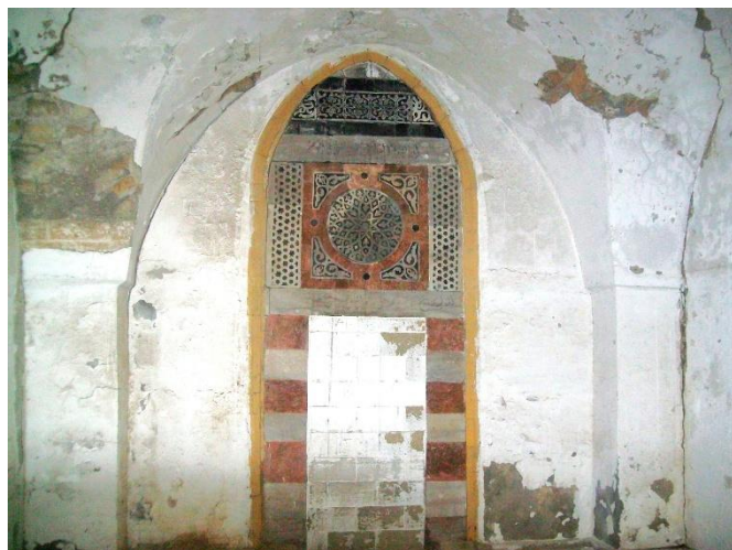
Fig. 4. Al-Ashi house, interior view of the Iwan Centre showing the decoration and the deteriorated plaster. (Source: Iwan Centre, 2011)
