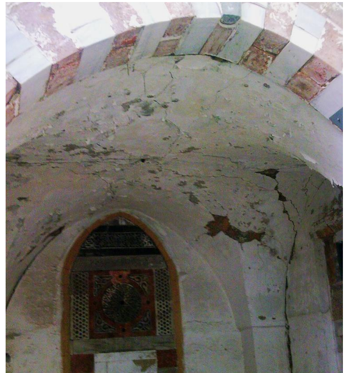
Fig. 7. Al-Ashi house, deterioration of the building and the effect of cement plaster. (Source: Iwan Centre, 2011)
