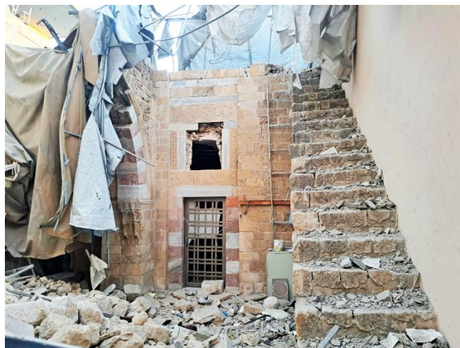
Fig. 14. Al-Ashi house, after bombardment. (Source: Iwan Centre, 2025)
