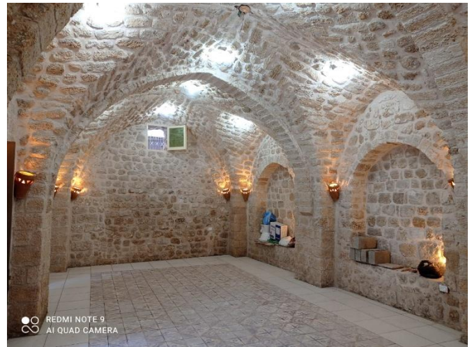
Fig. 11. Al-Ashi house, final treatment of stone walls and ceilings. (Source: Iwan Centre, 2021)
