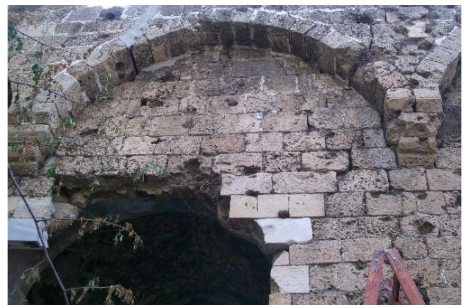
Fig. 4. Collapsing traditional houses in GOT. (Source: IWAN Centre, 2010)
