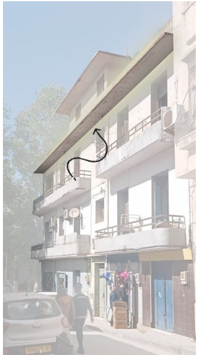
Fig. 26. An example of the concrete cap surrounding C typology facades. The concrete cap serves both aesthetic and functional purposes. It acts as a protective cover, preventing water from penetrating the top of the facade and causing damage. It also adds a finished, polished look to the building's exterior. (Source: Authors, 2024)
