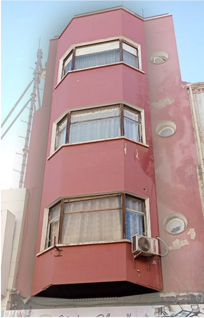
Fig. 18. A2b polygonal bow window type. A polygonal bow window is a type of window that extends outward from the main walls of a building, forming a shape with multiple flat segments, rather than a smooth curve. (Source: Authors, 2024)
