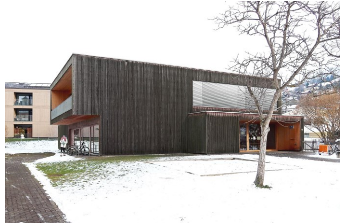
Fig. 12. A view of the ventilated facade, which has naturally changed to a grey shade due to weather exposure. (Photo: Jakub Hanták, 2023)
