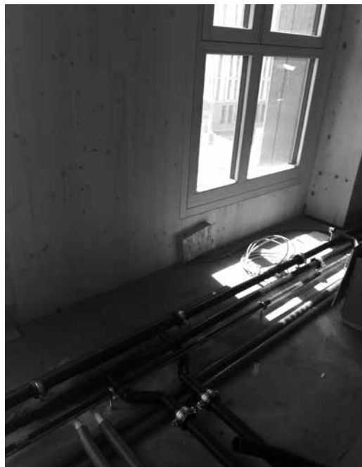
7 HoHo Vienna, technical installations on the floors Source: Darya Haroshka, 2018
